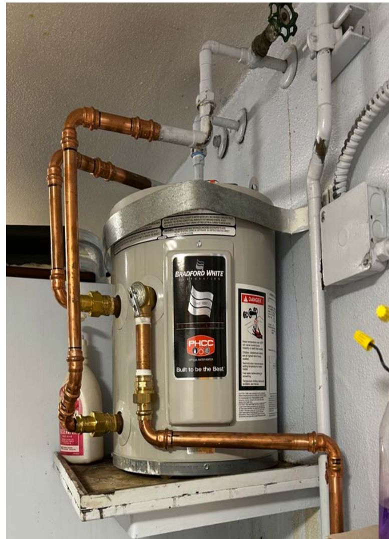
Fremont High School Bradford White - 6 gal. Utility 1.5kW 1 Element Residential Electric Water Heater Serial # WJ46527411
