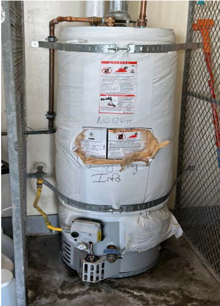
Madison Middle School Bradford White - FVIR Eco-Defender Safety System® 30 gal. Tall 32 MBH Residential Natural Gas Water Heater Serial # WH46461072
