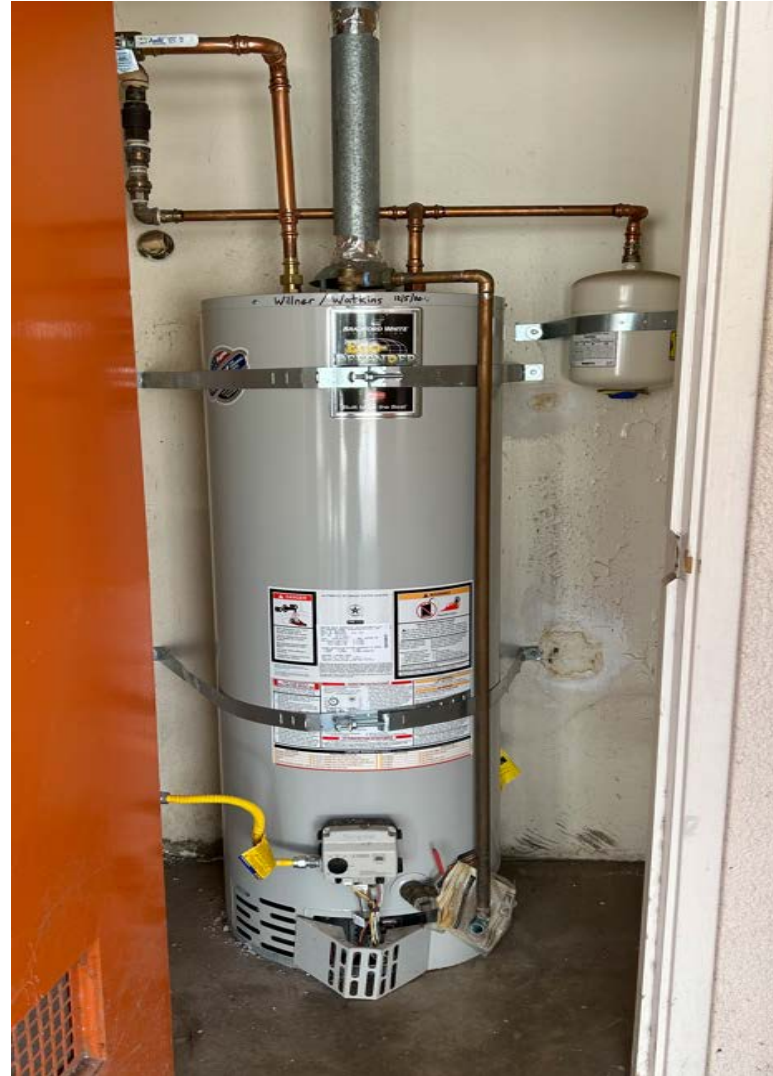
Vinedale Elementary School Bradford White - FVIR Eco-Defender Safety System® 40 gal. Tall 40 MBH Residential Natural Gas Water Heater Serial # WH46446612
