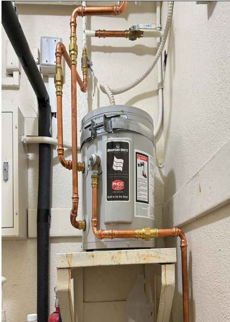
Franklin High School Bradford White - 6 gals. Utility 1.5kW 1 Element Residential Electric Water Heater Serial # XD47765629
