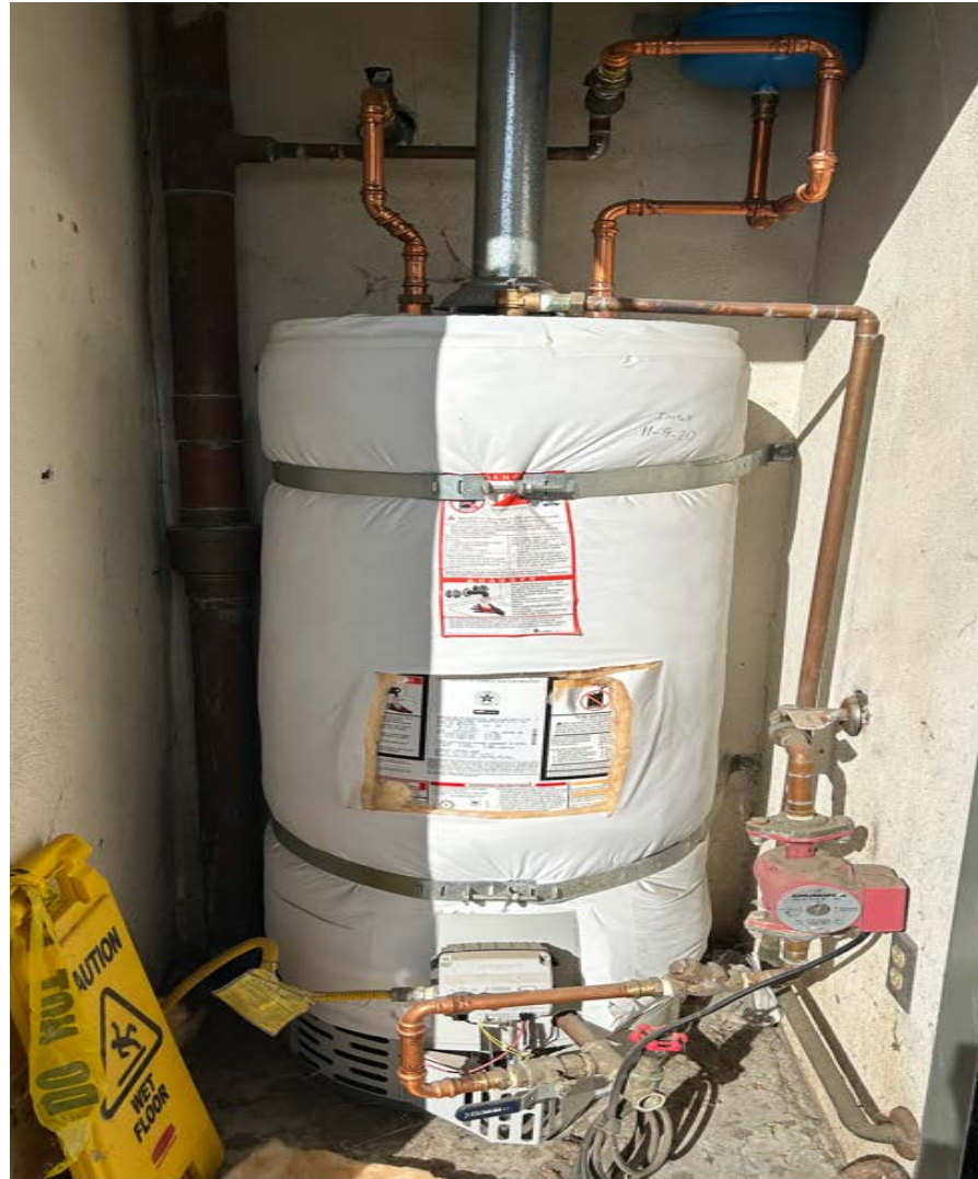
Mountain View Elementary School Bradford White - FVIR Eco-Defender Safety System® 40 gal. Tall 40 MBH Residential Natural Gas Water Heater Serial # WH46446624
