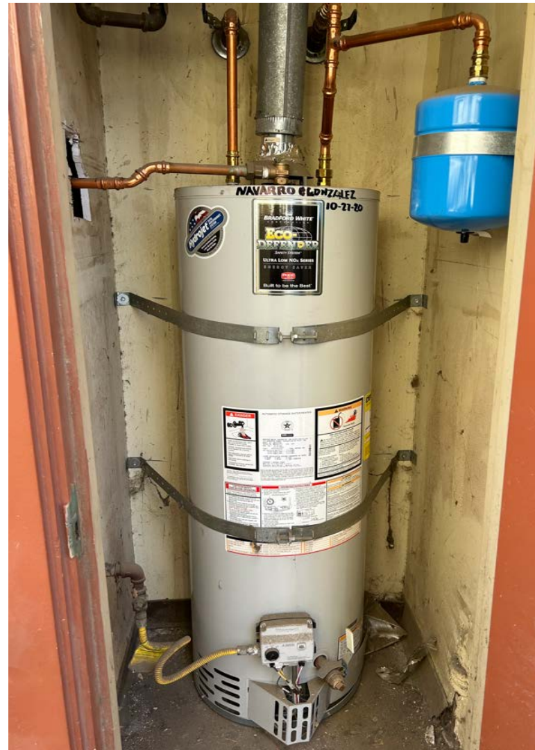
Olive Vista Middle School Bradford White - FVIR Eco-Defender Safety System® 30 gal. Tall 32 MBH Residential Natural Gas Water Heater Serial # WH46461070
