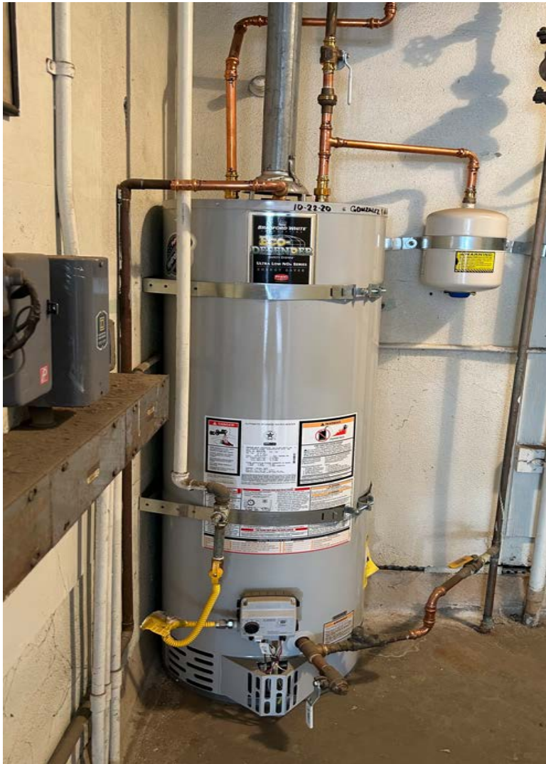
Olive Vista Middle School Bradford White - FVIR Eco-Defender Safety System® 40 gal. Tall 40 MBH Residential Natural Gas Water Heater Serial # WH46446608
