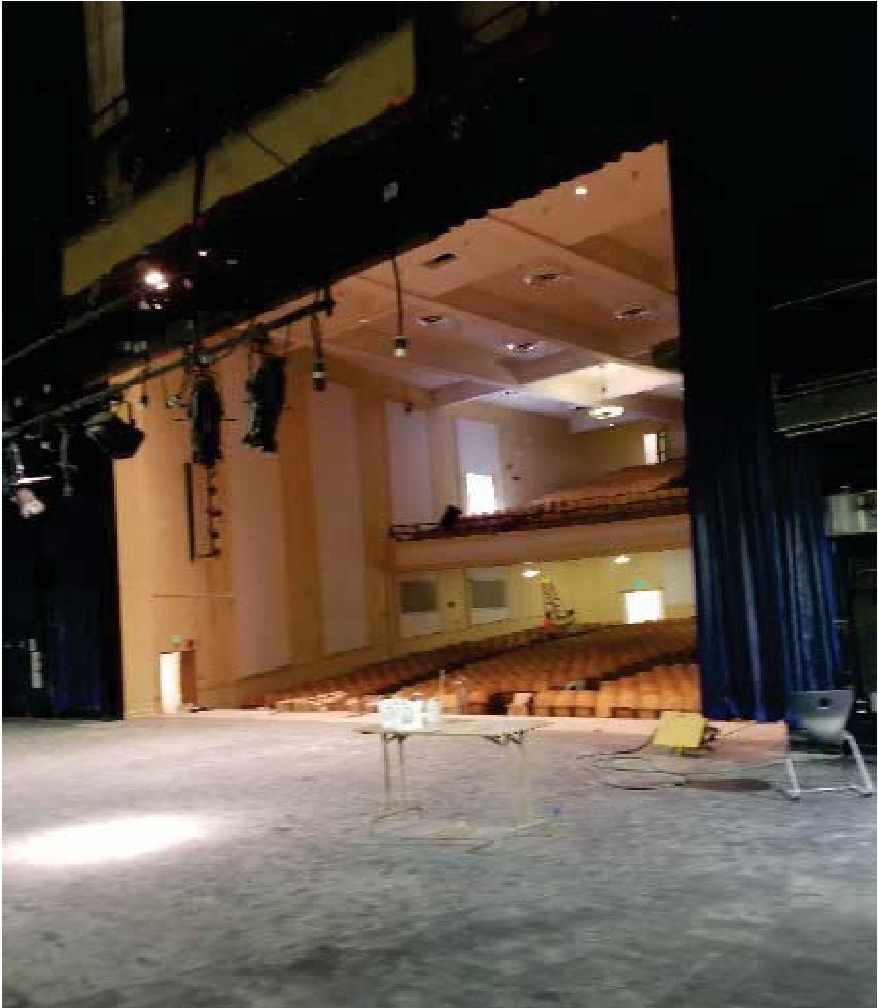
Renovation of the interior of the Auditorium Showing the Main Stage and 1 st and 2 nd Levels
