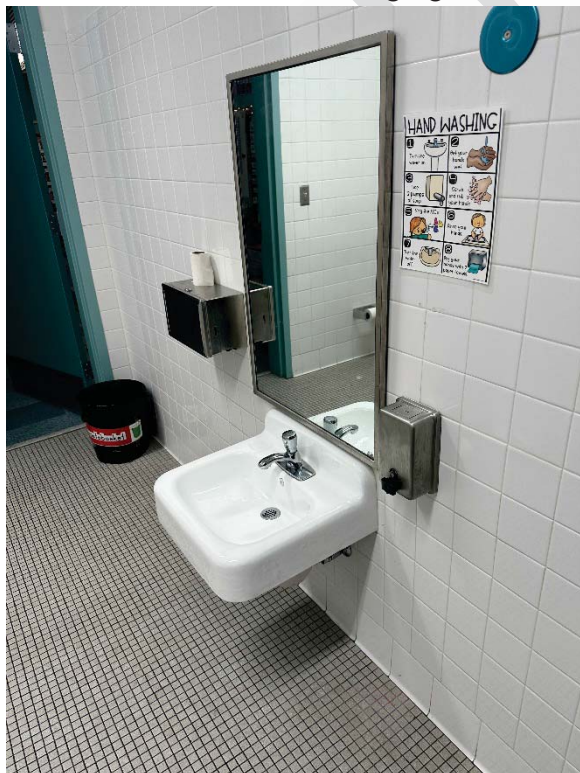
ADA compliant sink
