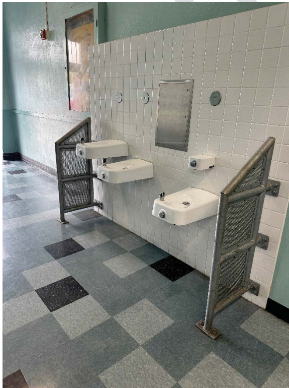
Indoor drinking fountains and railings
