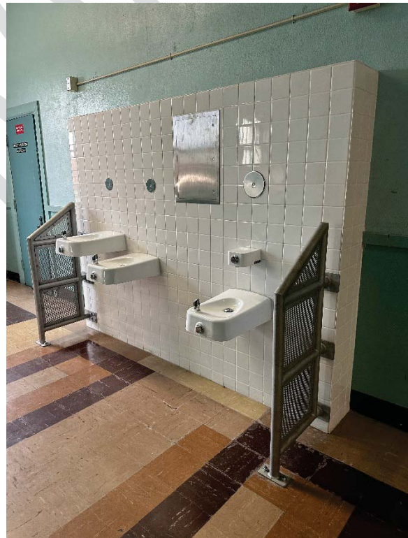
Indoor drinking fountains and railings
